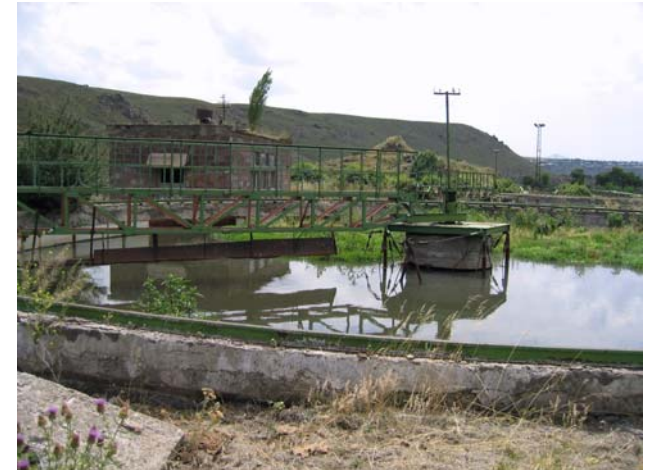
Armenian Wastewater Treatment Plant – Before Reform (2004)
