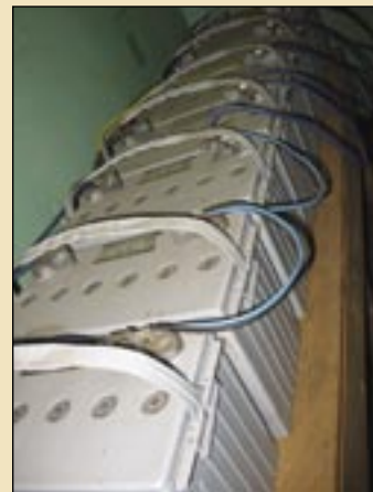
Battery banks provide additional power during surges and outages.
