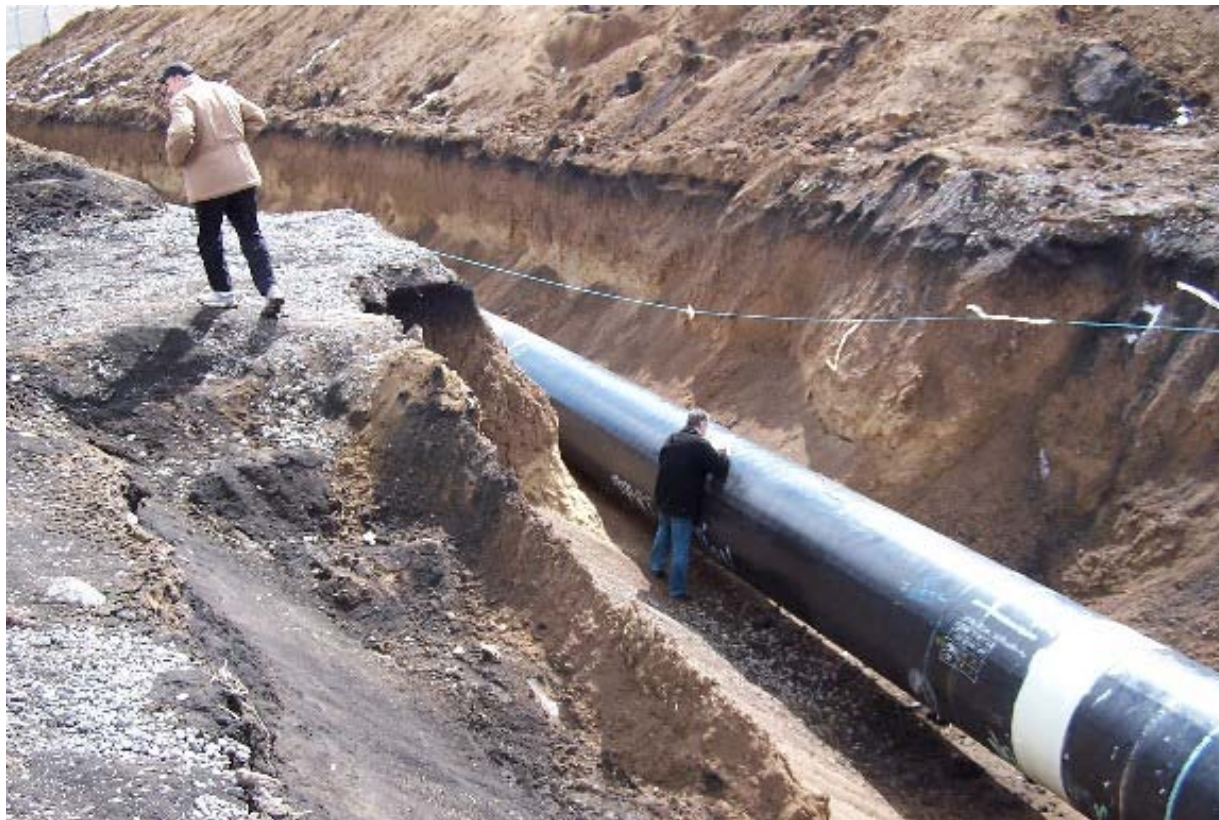
The Baku (Azerbaijan) -Ceyhan (Turkey) pipeline, (Picture from the Samtskhe Javakheti region- Georgia)
