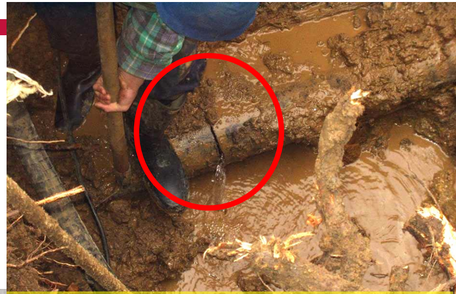
Broken secondary pipe, Romania
