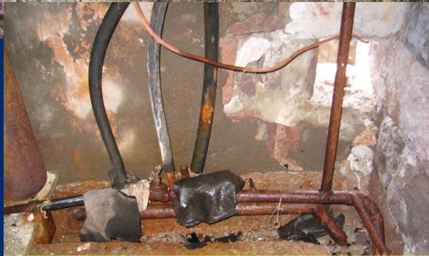
Corroded pipes, chlorination station, Armenia
