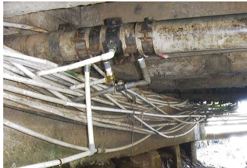
Illegal water connections in Indonesia
