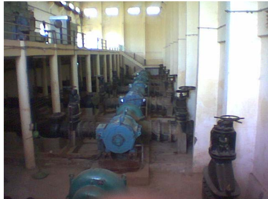
Pump room in Armenia
